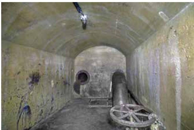
Fuel pipe inlets to Tank no. 5
